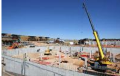
Construction is well underway in Newpark for a Best Buy store and a bowling alley.
